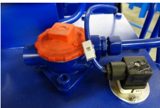
Fig. 42: filter unit & low oil switch
