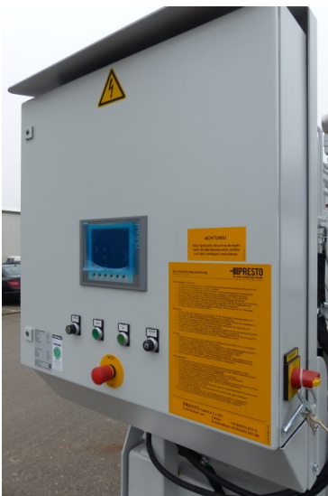
Fig. 67: switchgear box with operating controls
