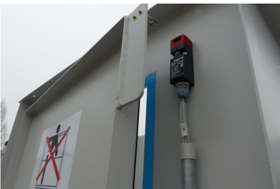
Fig. 17: safety switch inspection door
