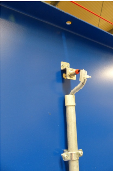
Fig. 82: light barrier level control
