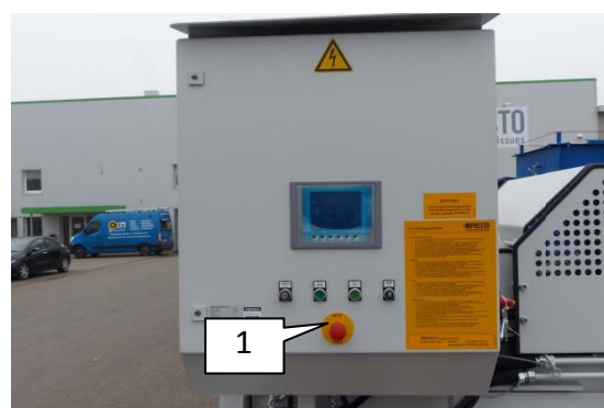
Fig. 8: emergency-stop switch, switchgear box
