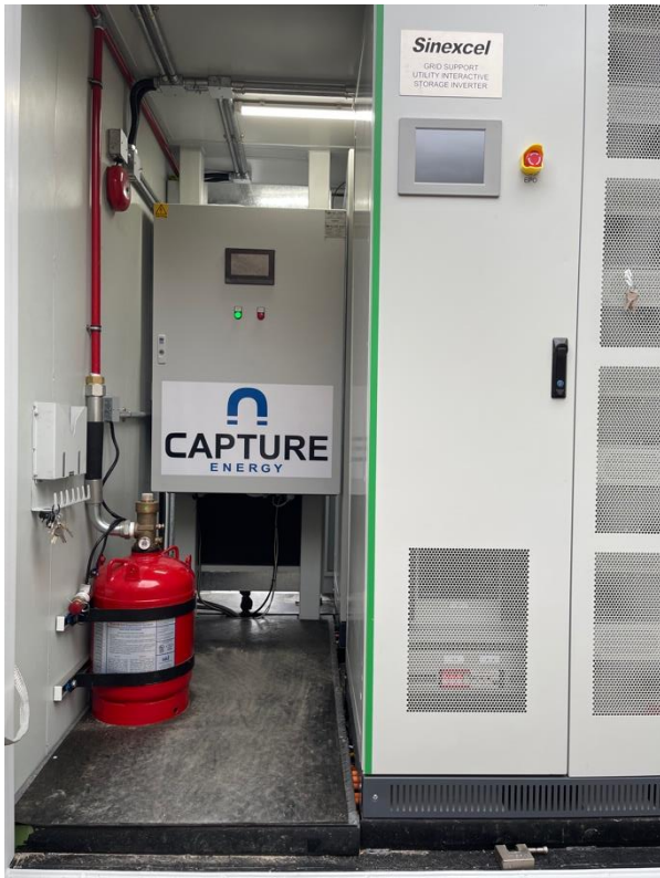
Figure 3: Picture of the first generation Capture Controller (with Capture Energy logo) inside a 1 MW/1.1 MWh container.
