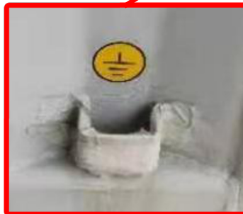
Container grounding point
