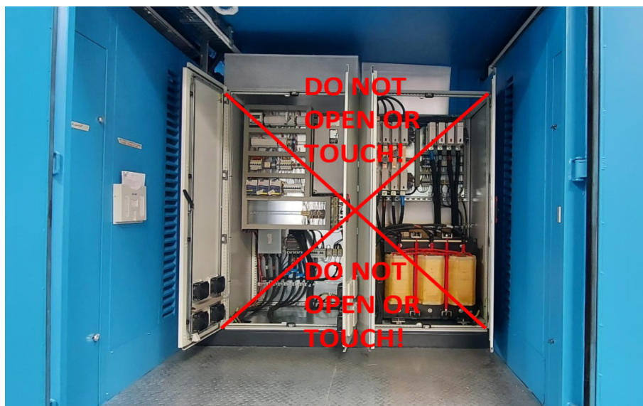
Figure 17: Power electronics inside Unlimited M20
