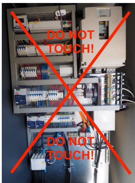
Figure 16: Power electronics inside Unlimited M10
