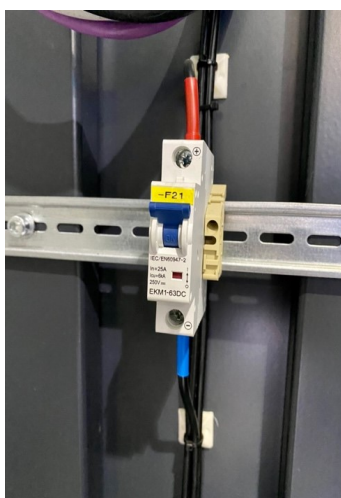
Figure 19: Circuit-breaker (battery cabinet)
