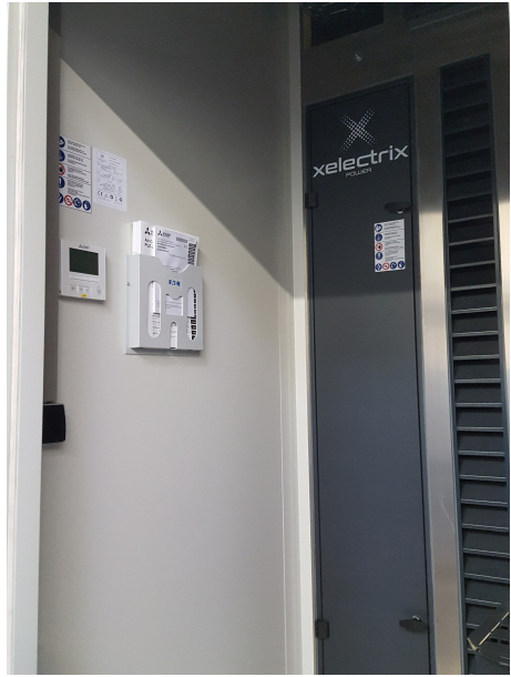
Figure 5: Warning label and nameplate inside the Unlimited Ranges
