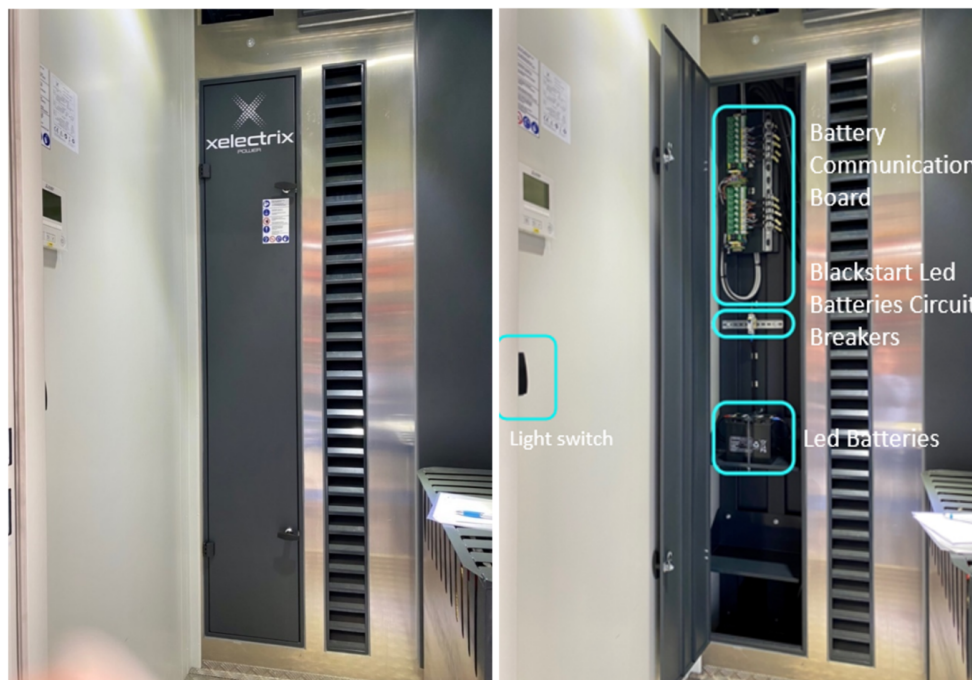
Figure 10: Battery control cabinet (communication system, circuit-breaker, black start batteries and light switch)
