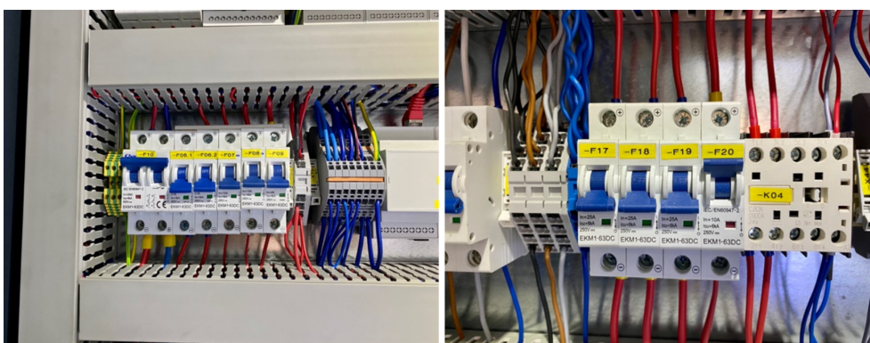
Figure 18: Circuit-breakers F10 and F20
